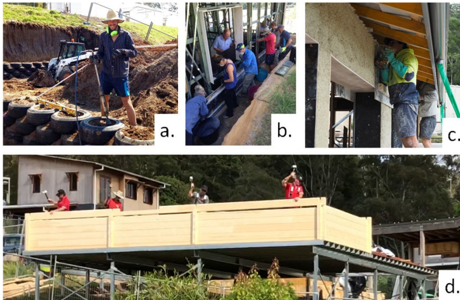
Figure 3 - Building technologies of homes 1 to 4. a. Compacting earth in tyres -earthship home 1 (Source: S. Bozkewycz); b. Home 2 volunteer hempcrete wall workshop (Source: G. Cameron); c. Home 3 hemp walls by builders (Source: M. Ong); d. Home 4 builders hammering together the solid timber wall (Source: P. Atkins)
